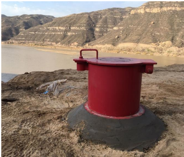
A groundwater monitoring well sitting on top of a mountain beside yellow river.
